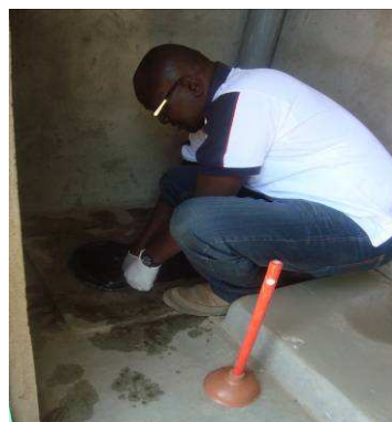
Fig. 7: ROSA project staff unblocking urine pipes at Daraja II primary school UDDT.
